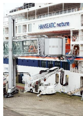
Shore power connection HANSEATIC nature
